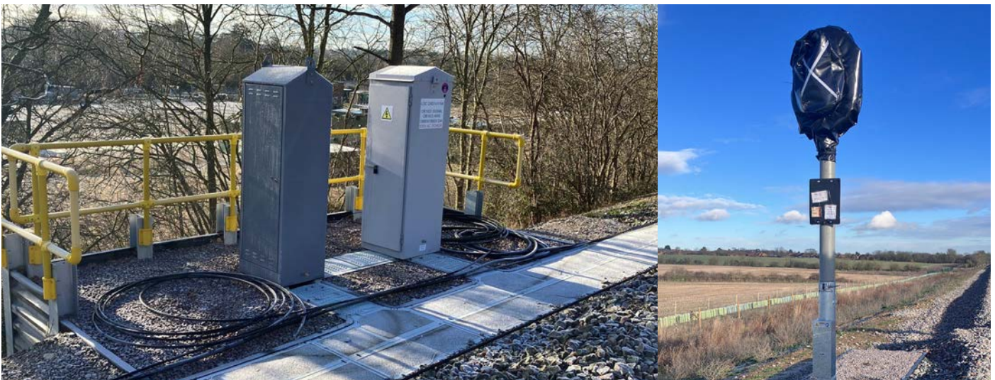
SPC cabinet equipment (left) and SPC line side signal (right).
